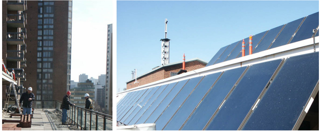
Solar panels are installed on the rooftop of Loretto College, Toronto, Ontario
