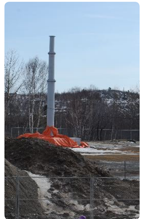
Construction starts on the new wind turbine at Walden Public School, Lively ON
